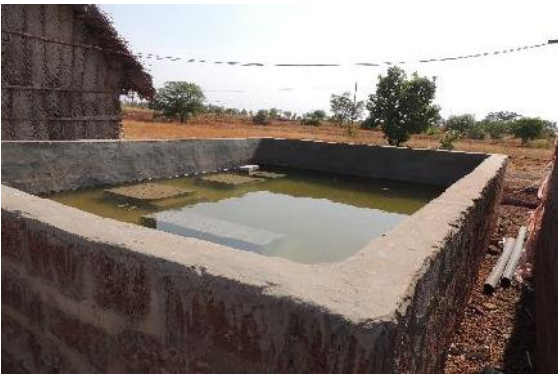
Photo 6-5: water tank for washing and domestic purpose
