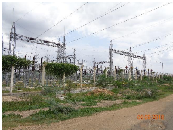
Pic 4-12: Grid sud station near Wadgera Village
