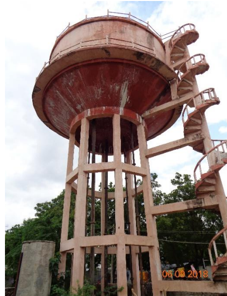
Pic 4-8: Water Tank
