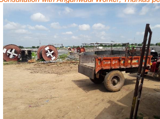
Chitapur 20 MW Solar Power Project site
