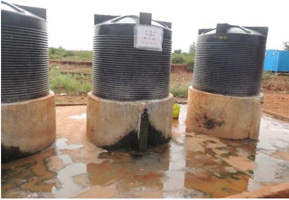
Tanks for drinking water consumption at Labor Camp, Chiknayakanhalli
