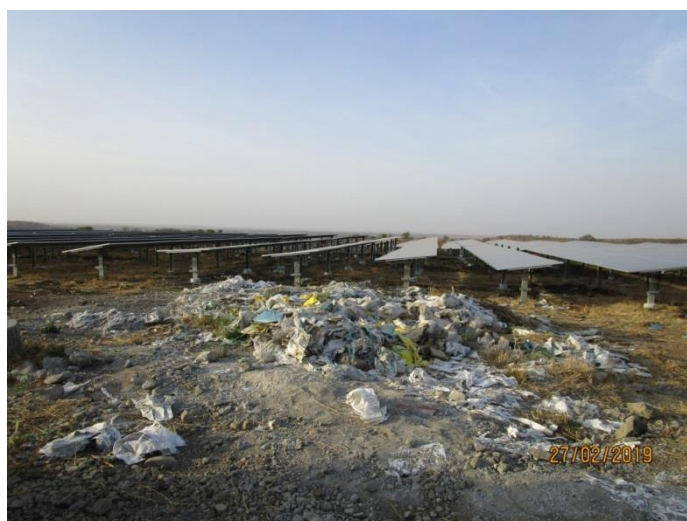
Construction waste dumped at the site
