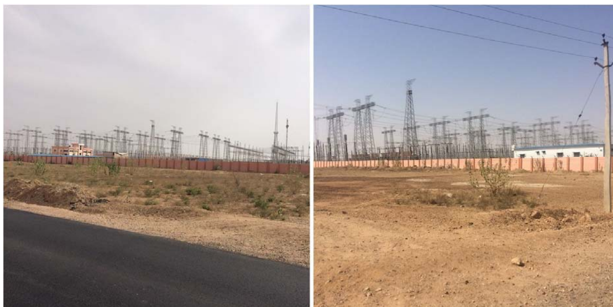
Figure 2.5 PGCIL 765 kV Grid Substation
